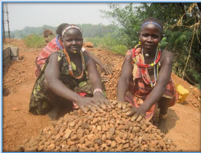
Figure 1 Toposa Women do most of the manual labor such as collection and sorting of stones for construction projects
